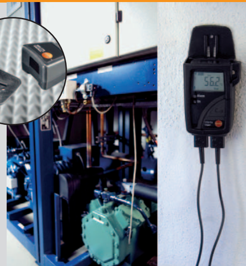
Measurement of air inlet and outlet temperature in refrigeration units
